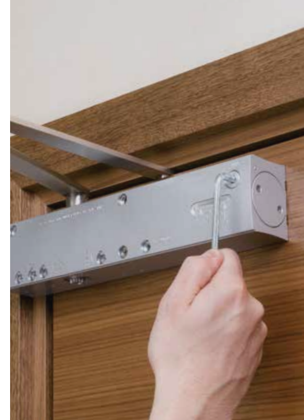
Door closer maintenance
