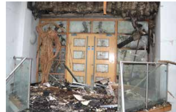
External side of fire door after fire
