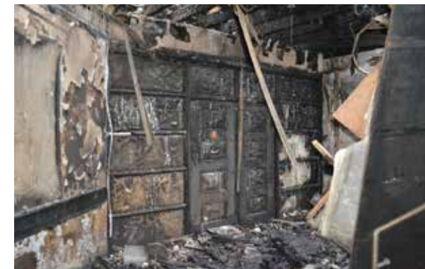
Internal side of fire door after fire
